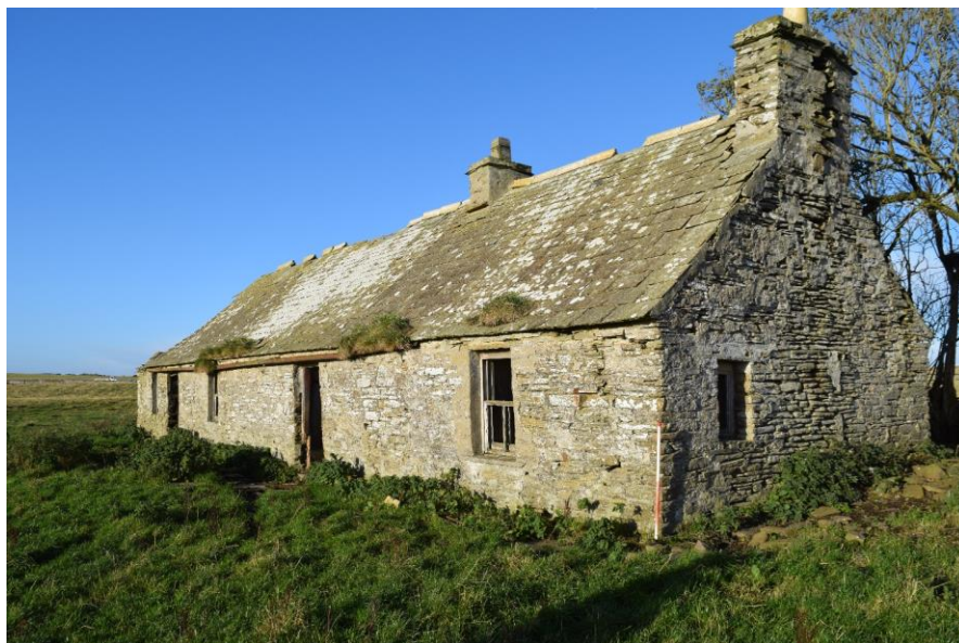
Figure 13-20 Derelict farmhouse at Skinnet (ORCA 69)
